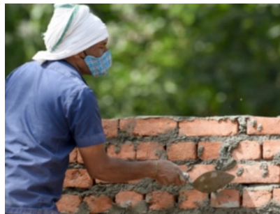
The state RERA bodies are trying to act strictly but are not able to do so because of restrictions in power.
